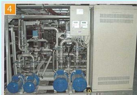
4 converter water cooling system
