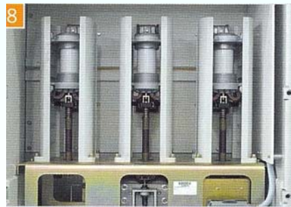
8 20 kV vacuum contactor output switch gear
