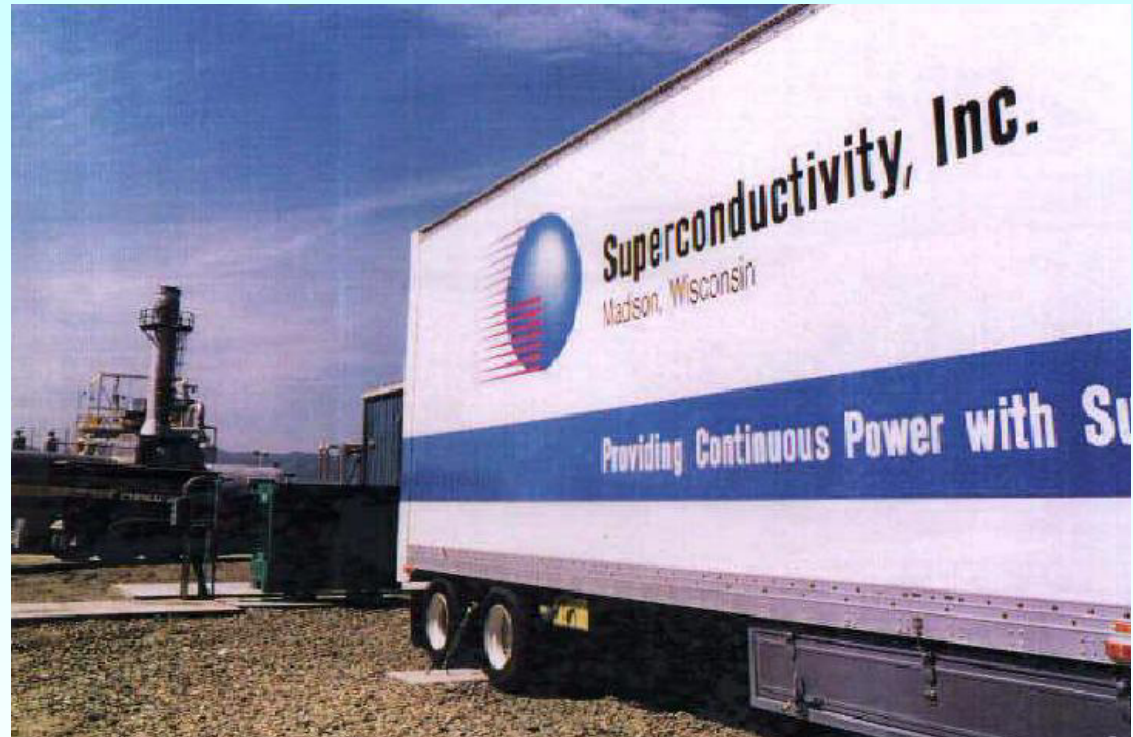
Installation of the complete SMES system ( S uperconducting m agnetic e nergy s torage) built in a container
