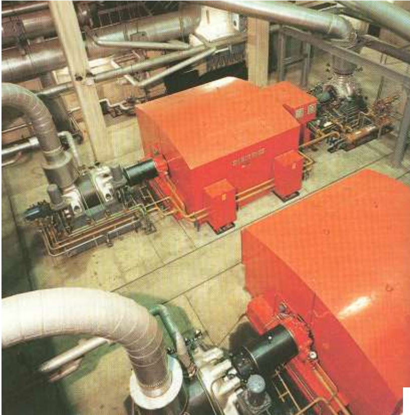
Feeder pump motors for thermal power plant boiler 15.1 MW at 5100/min
