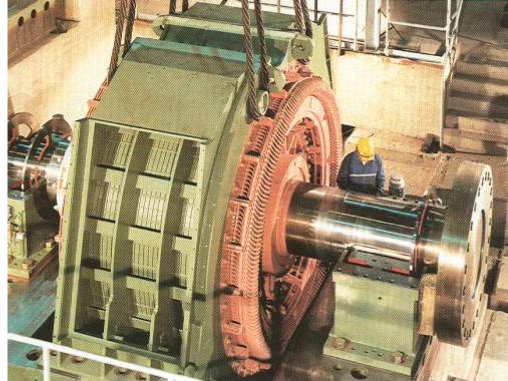
Main drive of 5.5 m rig of cold strip mill (1 st stage of milling process)
