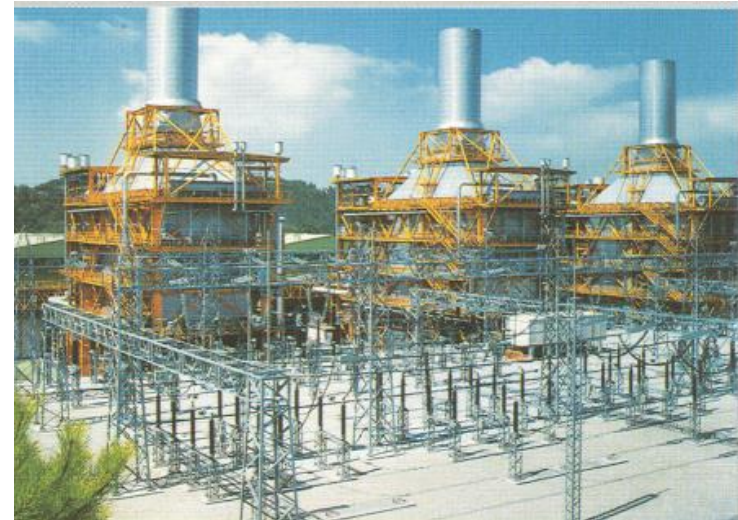
Combined cycle power plant (Gas and steam turbine process), Tapada do Outeiro, Portugal, Gas and steam turbine on a single shaft, 3 x 333 MW = 1000 MW
