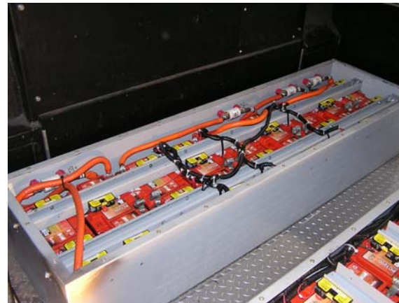
VRLA Vehicle Battery Pack String
